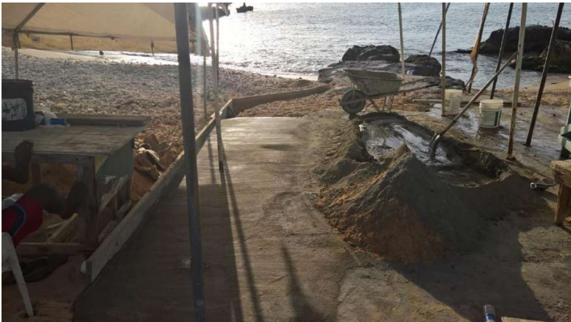
Image: Concrete slabs being made on the beach (Jan 2016) by the men at the Fish Market without permission from planning or the authorities. Illegal construction such as this has been done several times and it's worried that such works have caused damage to the beach and its environment. The landowner contacted planning immediately and discussed the matter with Ron S., he said it's the landowners liability / responsibility to stop such construction and planning couldn't do anything about it. Planning couldn't halt the works.
