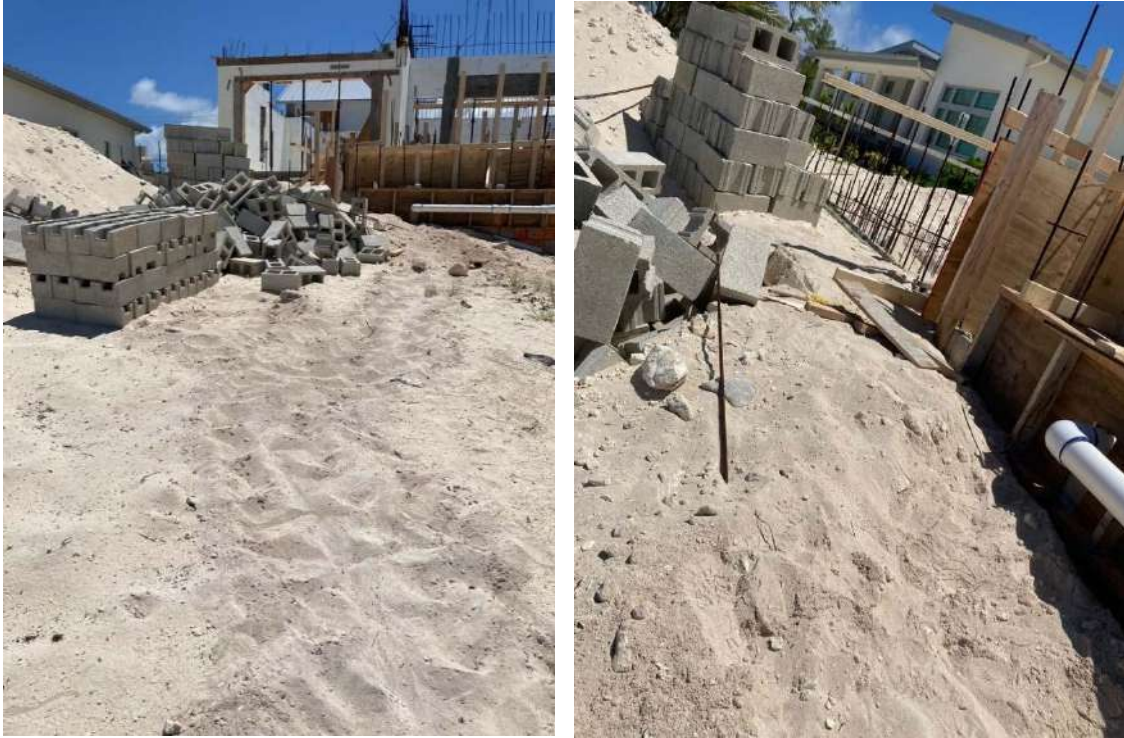
Figures 4 & 5: DoE photos showing turtle tracks within a construction site on a turtle nesting beach. This site did not have temporary beachside construction fencing to prevent turtles from entering the site. The turtle could have or may have been injured by construction materials and debris on-site (Source: DoE, 2023).
