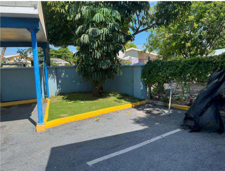
Figure 4: The existing concrete wall and damaged chain link fence at Elizabethan Square.
