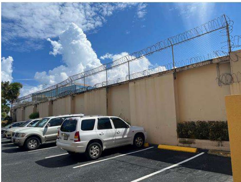
Figure 2: Barbed wire and razor wire above the wall and chain link fence at the George Town Police Station.
