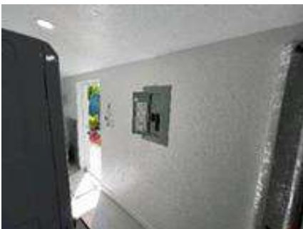
Electrical Panel Box in ATF Unit
