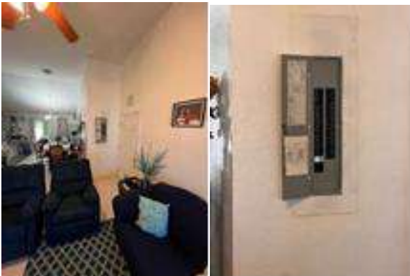
Electrical Panel Box in Main Unit
