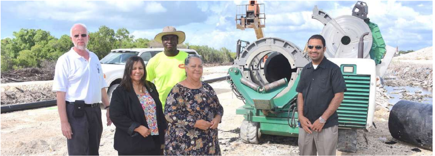
(From left-to-right) Water Authority's Deputy Director-Tom van Zanten and Director-Dr. Gelia Frederick van-Genderen, Hon. Juliana O'Connor-Connolly and ACO Wilbur Welcome conduct site visit to inspect infrastructural works.
