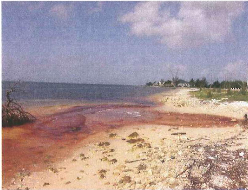
Fig 5: Red tannin stained water flowing into South Sound at the present culvert (2008).
