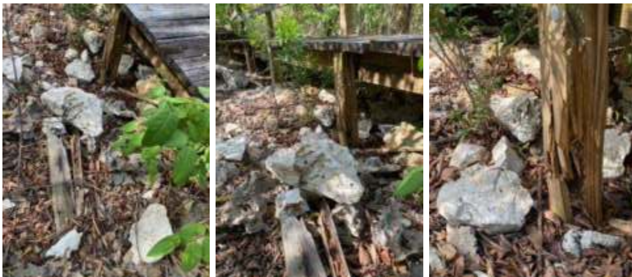
Figures 4-6: DoE site visit photos showing fly rock from the West End Quarry on the Salt Water Pond Trail and damage to the Salt Water Pond Trail boardwalk. (Source: DoE, taken: 30 March 2023)
