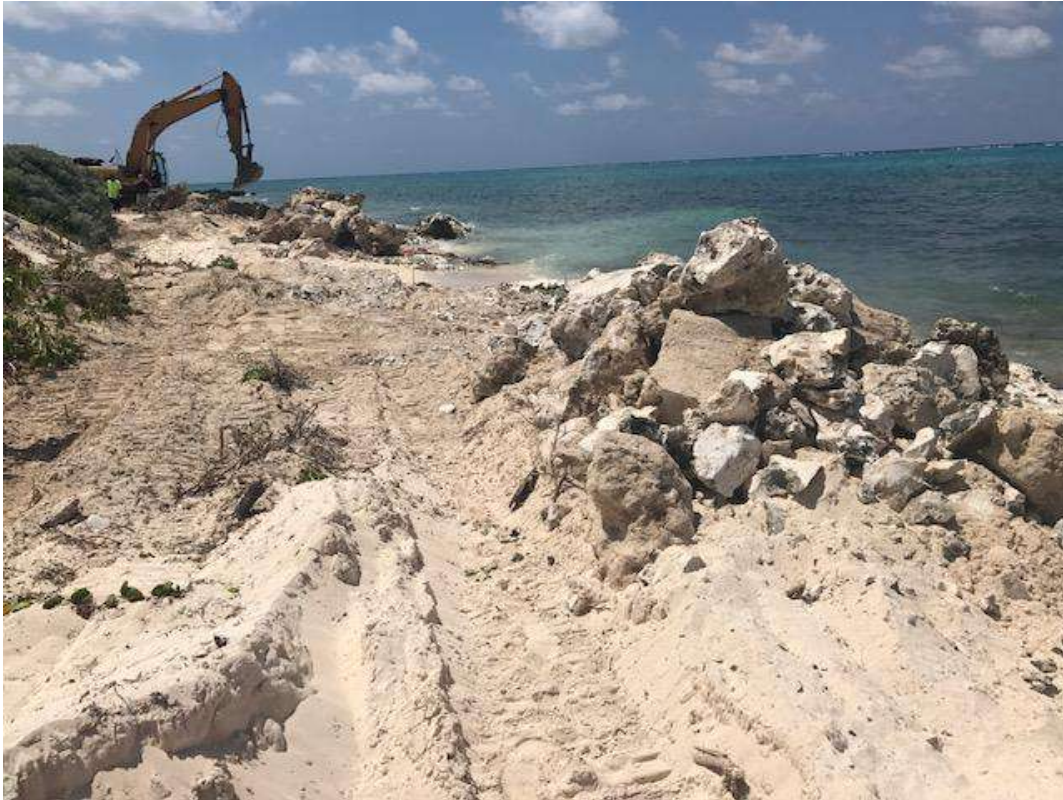
Figure 8. Stockpiling and on-land activities impacting the marine environment through turbidity and deposition of waste
