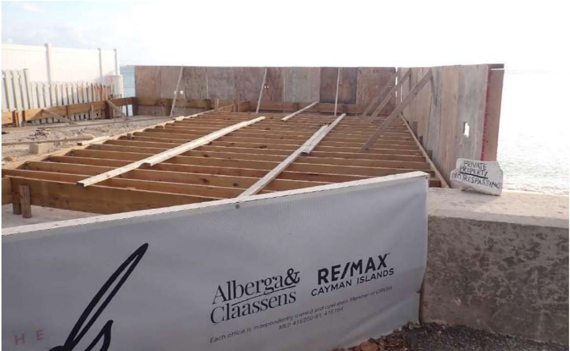
Figure 1. The site as of 7 December 2023 with a partially constructed deck (Source: DoE, 2023).
