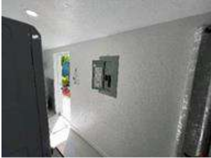
Electrical Panel Box in ATF Unit
