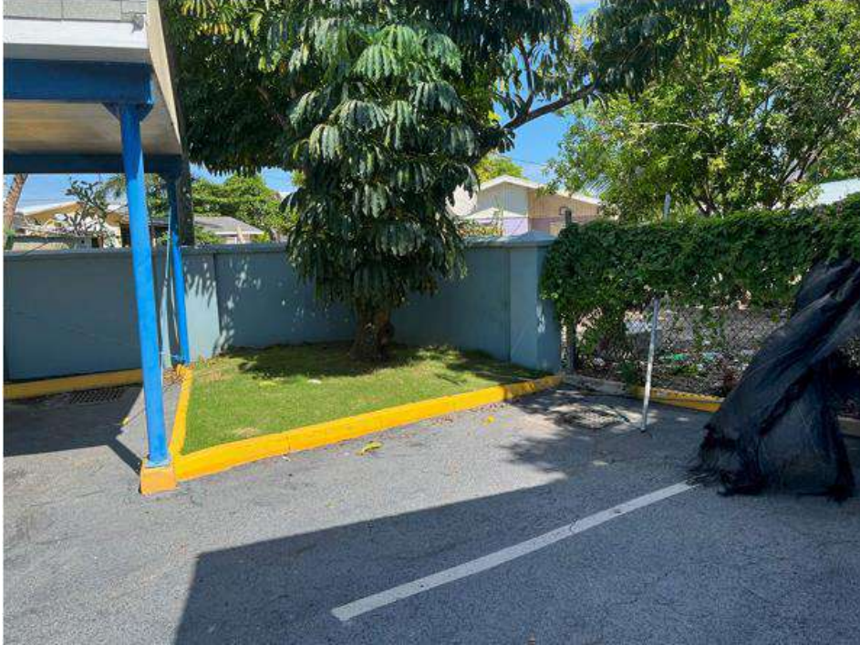
Figure 4: The existing concrete wall and damaged chain link fence at Elizabethan Square.
